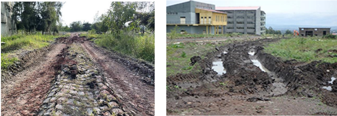
Figure 1: Collapsed cobblestone road section founded on unstable subgrade soil
